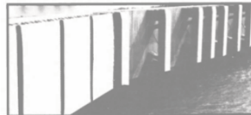
SOLIDUR fender facing on rail ferry terminals.
